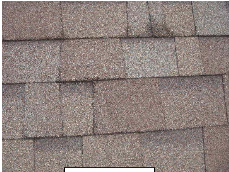
Roof surface worn, but in fair condition
